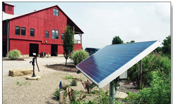
A solar panel located on the south side of the Westmoreland Conservation District headquarters powers a pump that moves water from a 3,000-gallon cistern uphill to help water flower, herb, and vegetable gardens maintained by Penn State Cooperative Extension.
