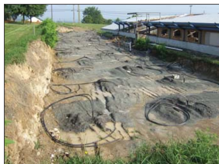
Geothermal wells at GreenForge with tubing in place and ready to be connected.
