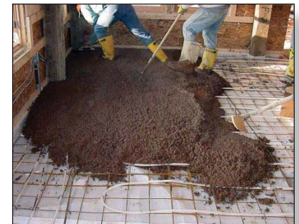
Concrete for flooring is poured over tubes that carry warm water from the geothermal system in the winter.
