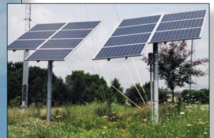
Penn State Cooperative Extension's wind turbine and solar array
