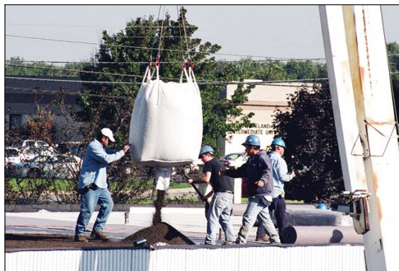
Cranes were used to lift the sacks of special planting media and distribute it over the surface of the GreenForge roof.
